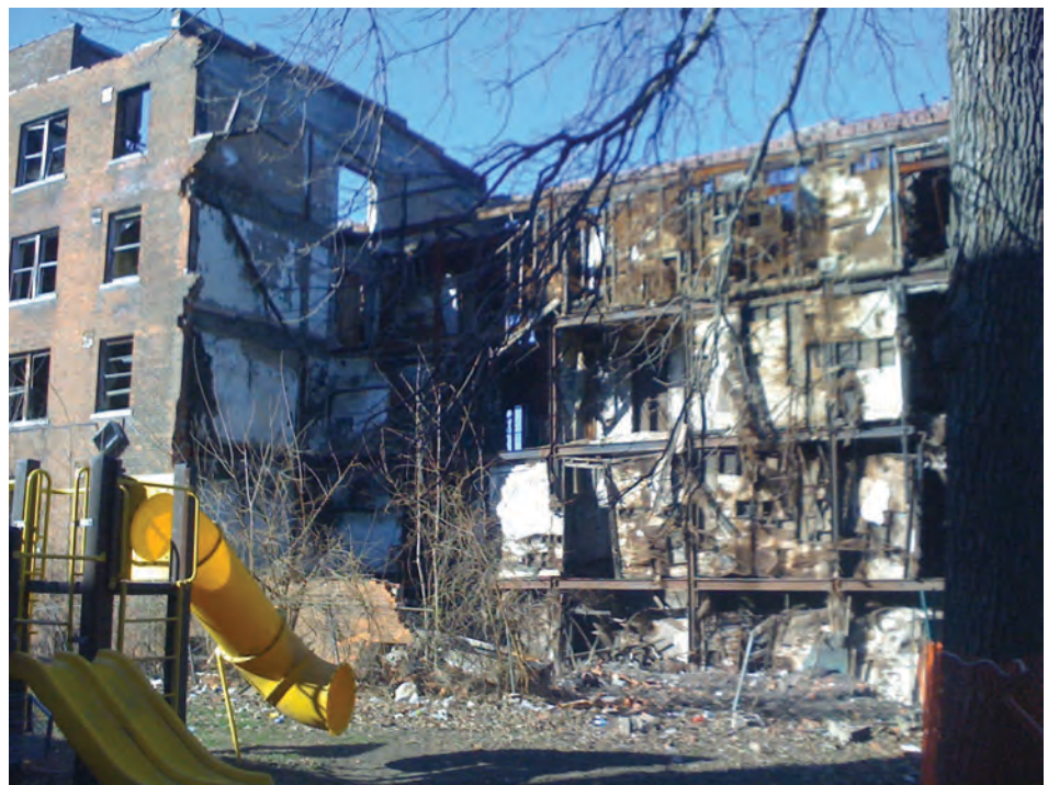
This abandoned building in Highland Park will be part of the demolition to create safer neighborhoods.
